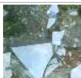
Broken window glass Cristal fracturado
